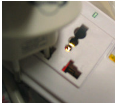
Exposed metal 'live' parts
